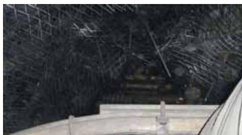
Manifestations of rock pressure in the mining entries: а – deformations in the form of roof sagging in the excavations supported by single-level roof bolts; б – roof doming in the excavations with combined support
